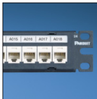
Patch Panel Labeling
