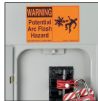
Safety Sign Labeling
